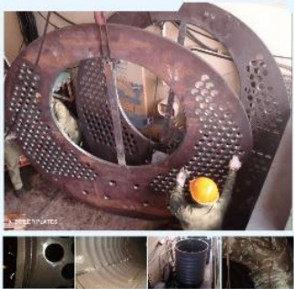
REPLACEMENT OF CORRUGATED FURNACE TUBE PLATES AND SMOKE TUBES POST-WELDING HEAT TREATMENT ON SITE
